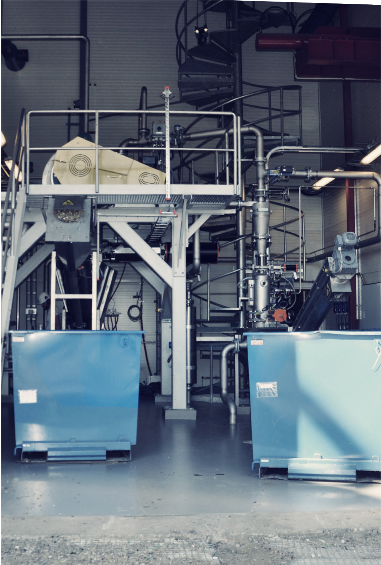
The equipment supplied by Cellwood Machinery is installed in a separate hall at Frevar KF Biogas Anlegg in Gamle Fredrikstad. The premises are neat and clean with hardly any odours. To the right of the picture: Separation of heavier particles such as glass, gravel, and metal. To the left of the picture: Separation of plastics.
