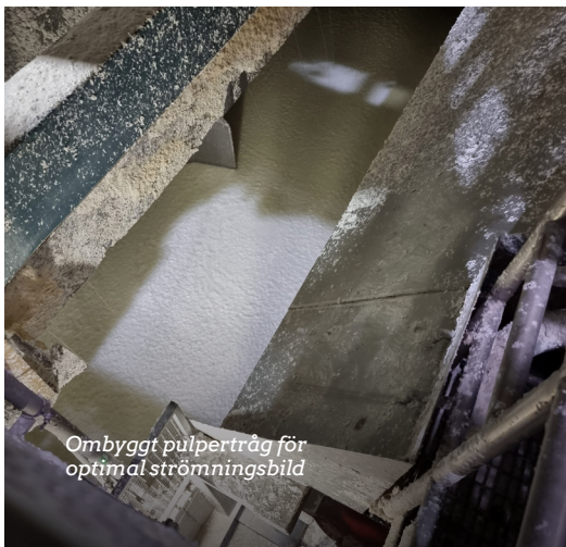
SCV Expansion 2.0 / Broke Handling
