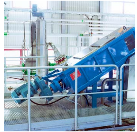
Thickening by inclined screw dewatering.
